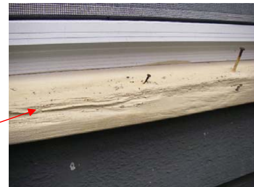
Samples of damaged exterior: Siding rot Rotten windowsill painted
