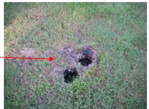
Pipes to be properly capped
